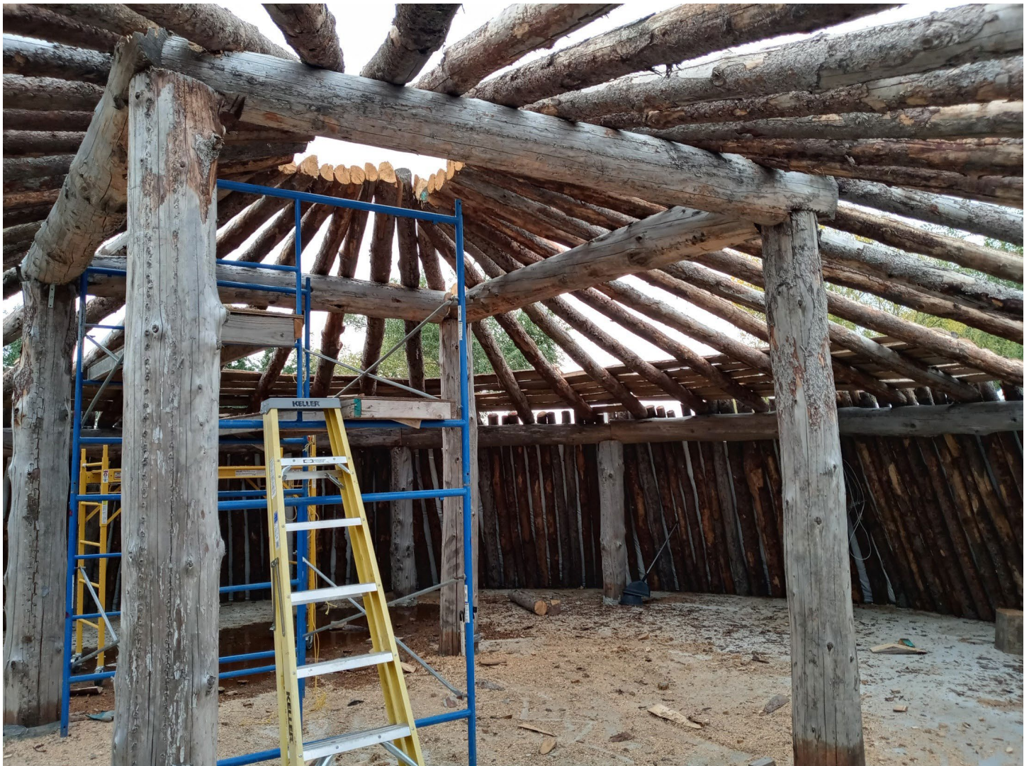
An earthlodge under construction at the Zani Otunwe site. Image courtesy of Waziyatawin.
