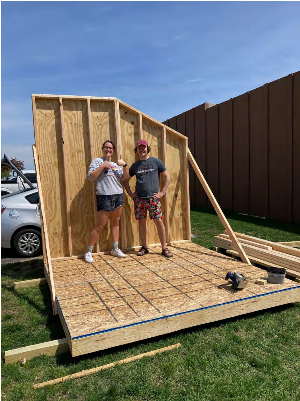
The floor and one wall of the solar shed as it is being framed. The shed sits on two four-by-four wooden beams. Image courtesy of Joseph Underhill.
