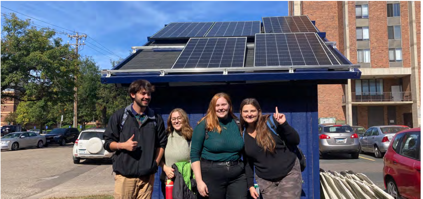
The solar shed is now fully painted and the solar panels are partially installed. Image courtesy of Joseph Underhill.
