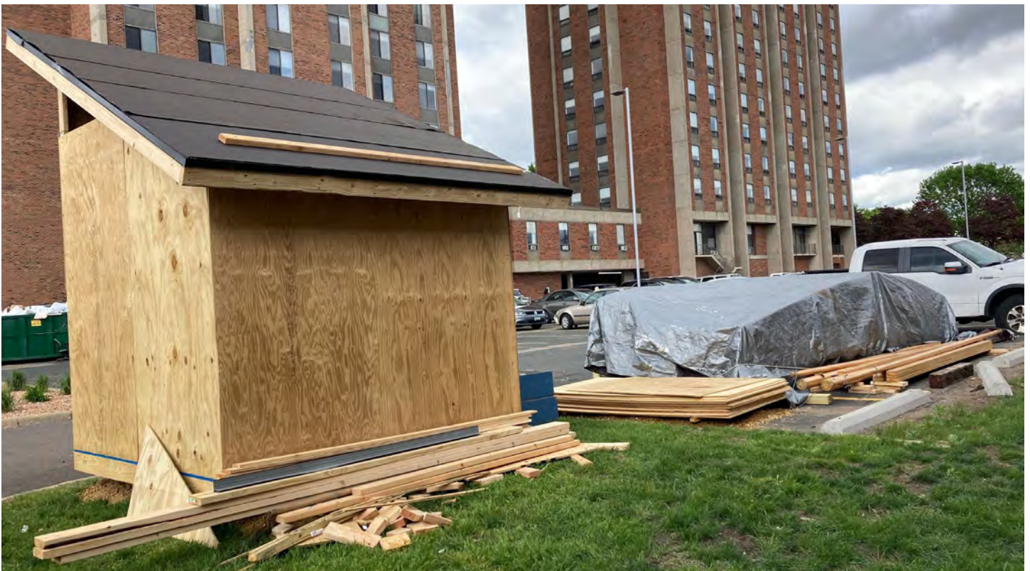
The solar shed, now framed and covered with tar paper on the roof, sits on the edge of a parking lot at Augsburg University. Image courtesy of Joseph Underhill.
